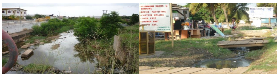
Poor State of Storm Drain near Spintex Road Choked Community Drain
