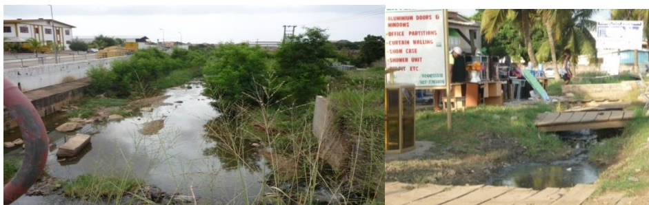
Plate 3: Poor State of Storm Drain near Spintex Road
